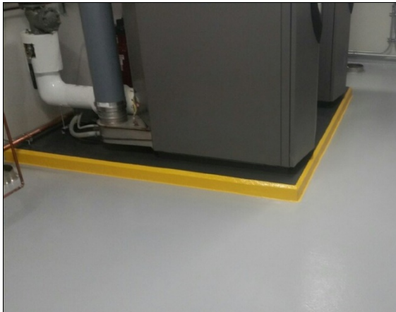
PHARMACEUTICAL FACILITY (FOR CHEMICAL PROTECTION)
