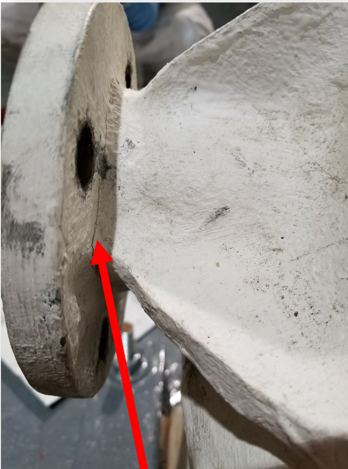
Small hair line crack at the flange to pipe transition.
